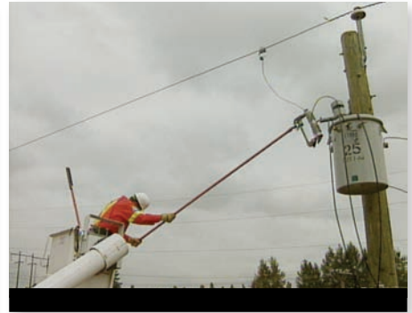
A typical shot of a line worker reclosing a re-fused cut-out. Without an IFD there is no way to know the consequences of this action.
