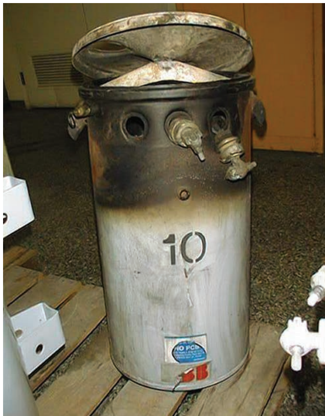
The force of an internal fault inverted the lid, which is still attached to the center post, causing a catastrophic failure.
