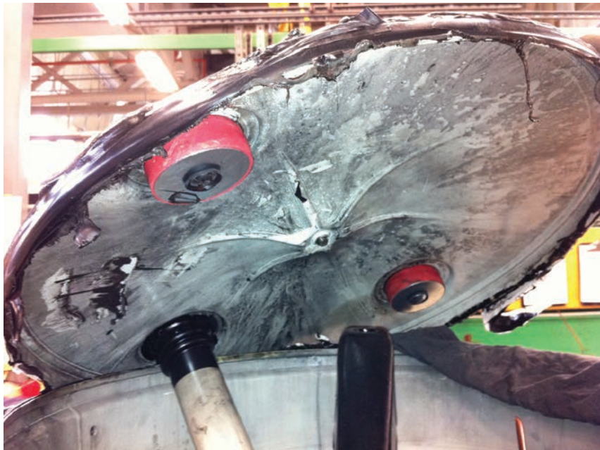
An internal fault can be violent enough to blow the lid off a transformer.
